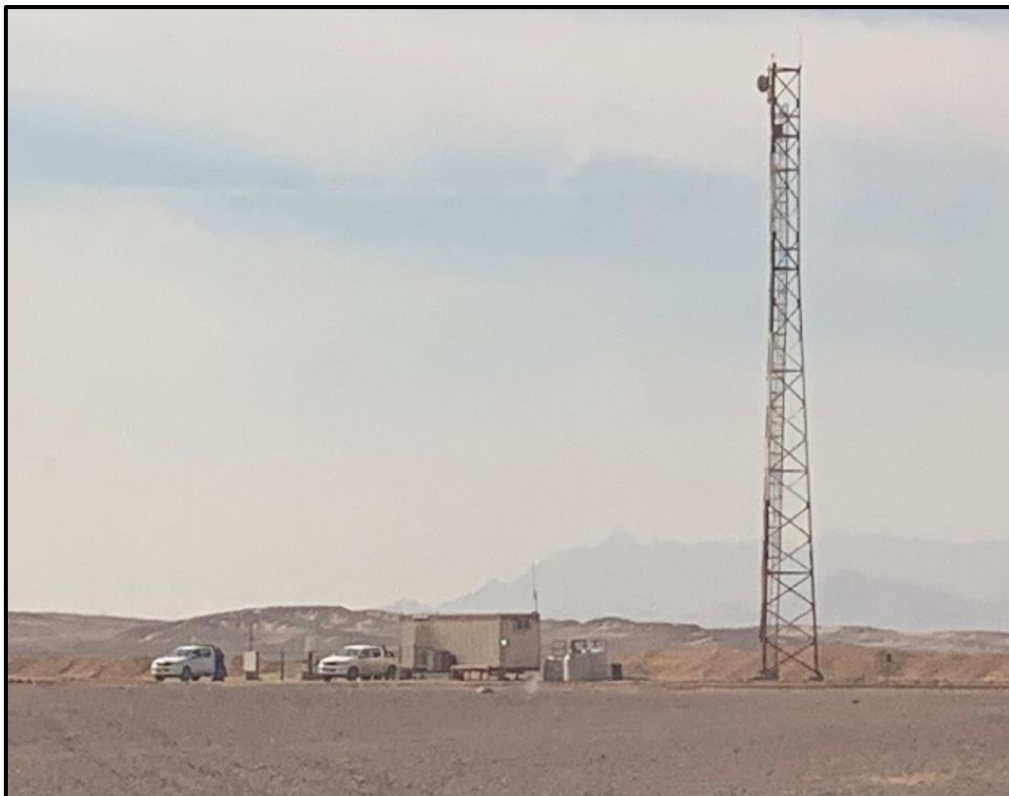
Figure 8-61: Telecommunication Tower within Petroleum Storage Facility Onsite
