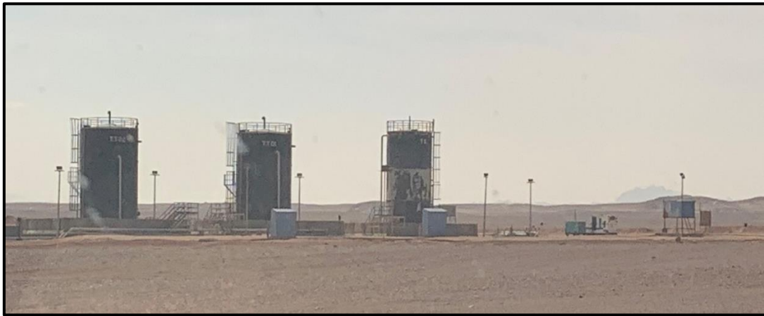
Figure 8-8: Petroleum Storage Facility
